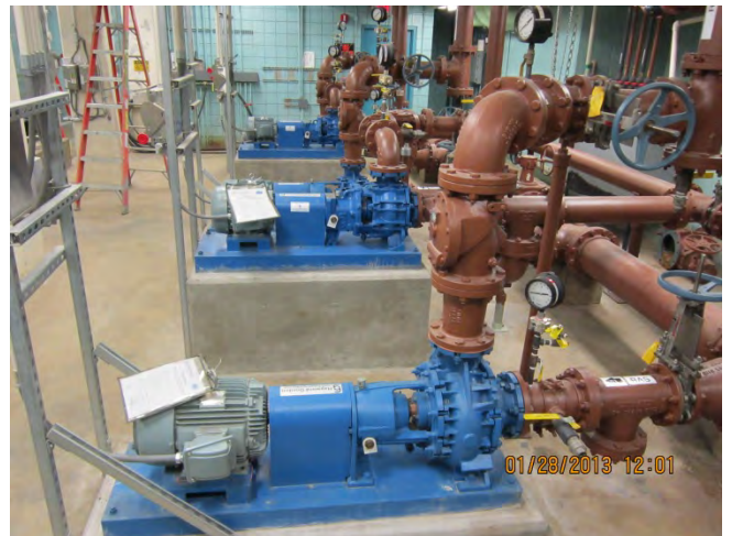
New RAS / WAS Sludge Pumps
