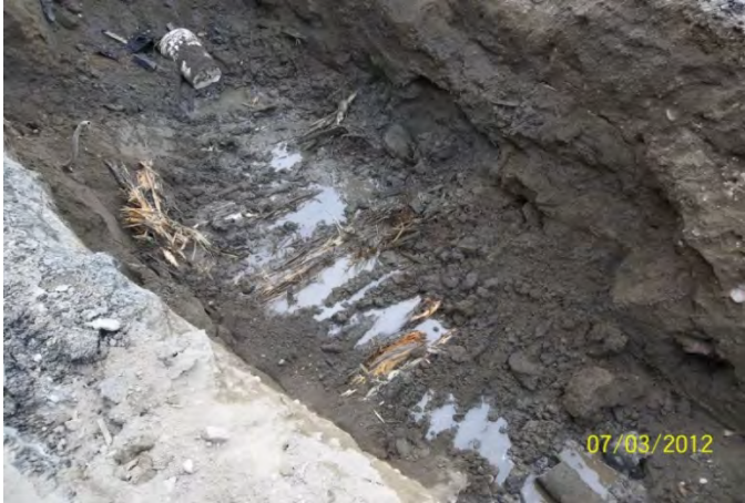
Old Wood Cribbing Under 1893 Pipe on Lebanon Street
