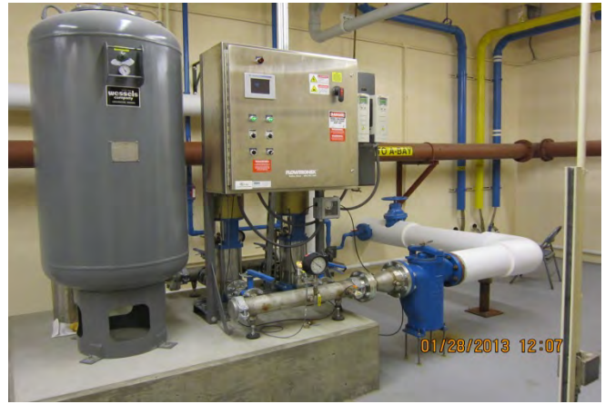
New Plant Water System
