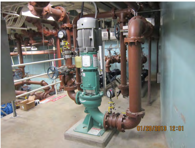
New Digester Recirculation and Transfer Pumps
