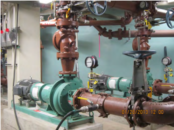
New Anaerobic Digester Mixing Pumps
