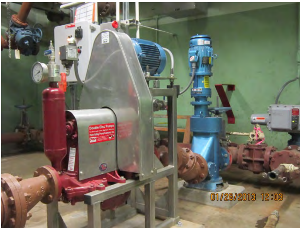
New Primary Sludge Pumps
