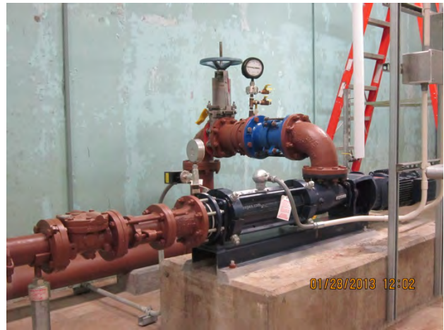
New Centrifuge Feed Pumps
