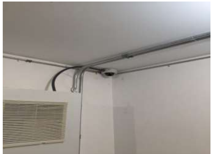
Security camera set up at the Greensboro Pump Station
