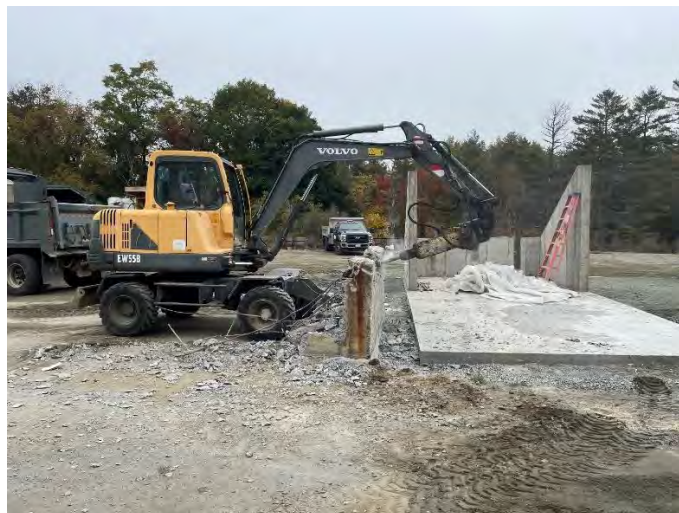
Photo showing the removal of a structure and the construction of the housing for the new grizzly
