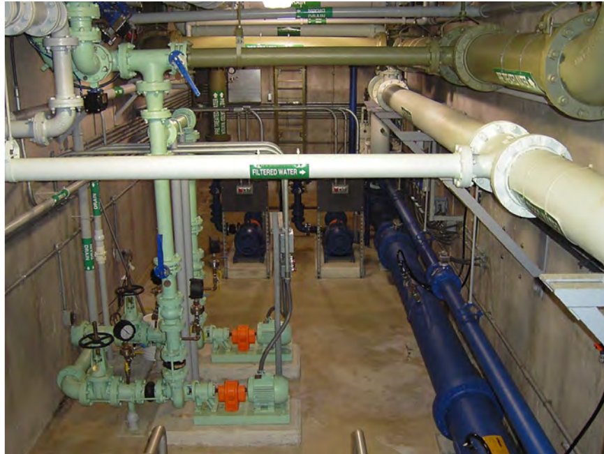
Water Treatment Facility Pipe Gallery
